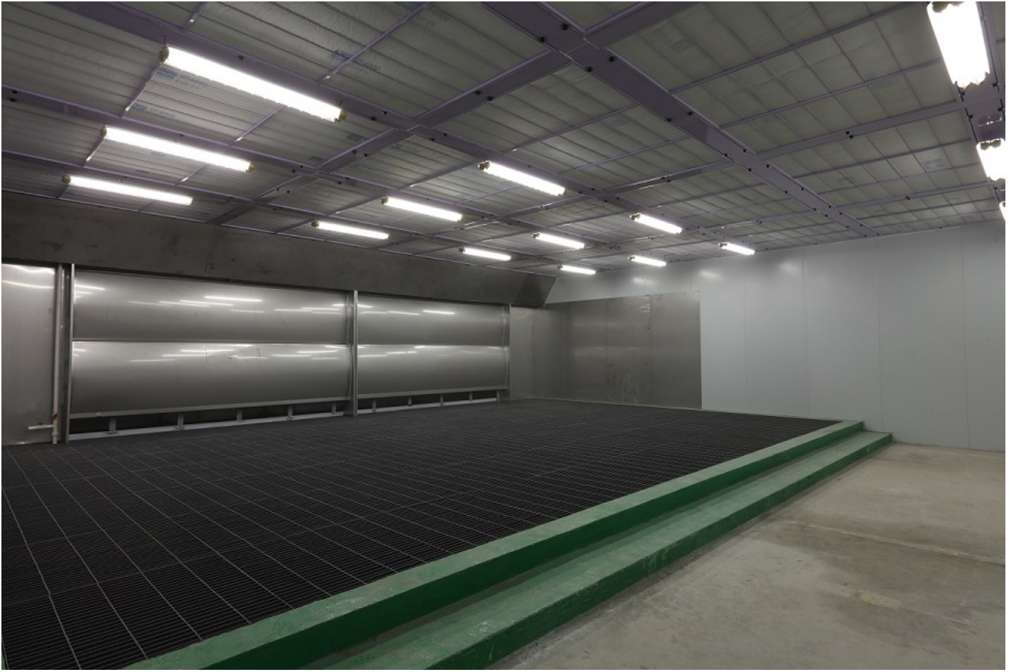
Painting workshop of the EHang Yunfu facility
