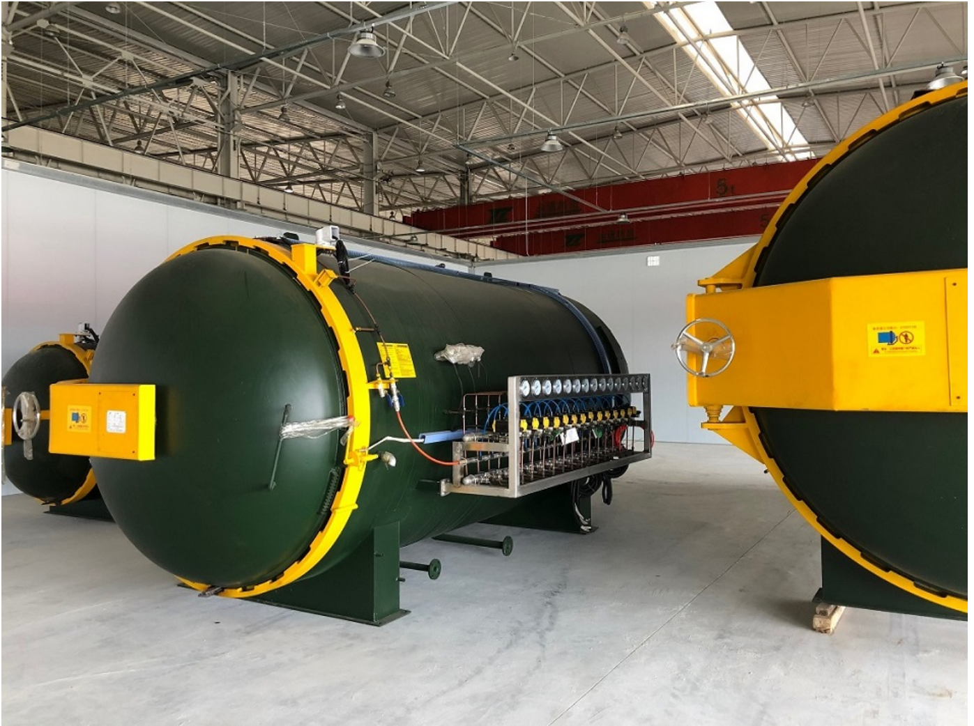
Autoclaves for various parts processing of the EHang Yunfu facility
